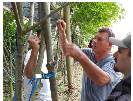
Welding of two tree shafts to form a cross brace under the "Growing Footbridge" in the botanical trial field in Kamen
