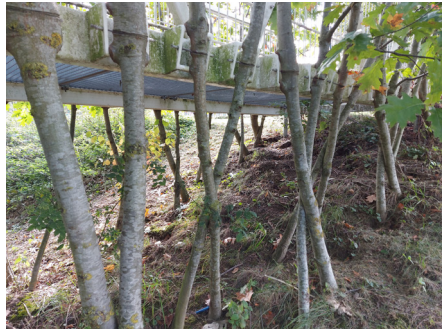
Young red oaks grow together with each other and with the bearing points of the footbridge to support it
